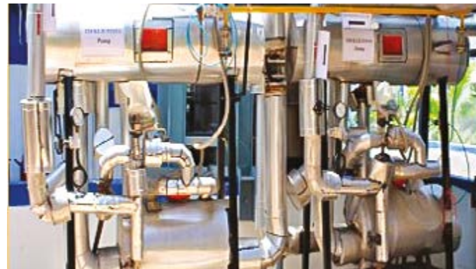
Installed packaged pressure powered pump unit (PPPPU)
