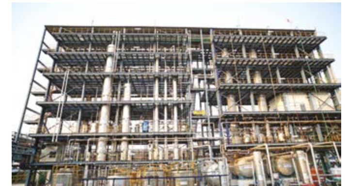
Solvent recovery system
