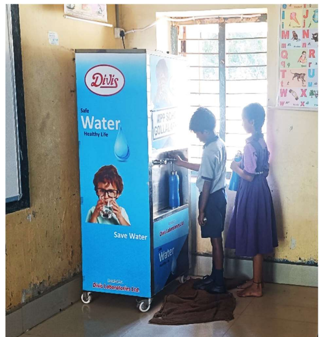
Pic 13 – RO unit inside a Classroom
