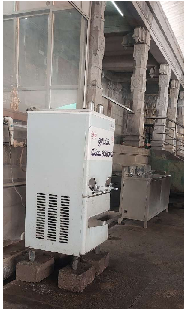
Pic 8 - Chiller & sink inside the temple
