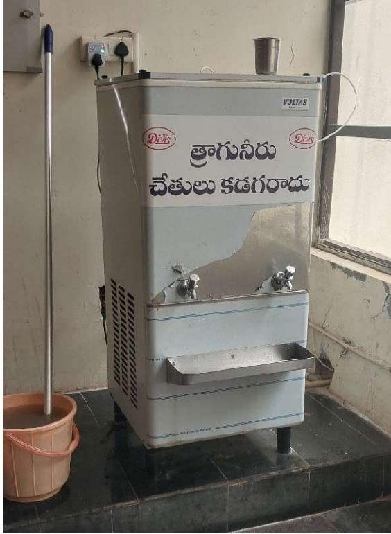
Pic 22 - Chiller in a guest house
