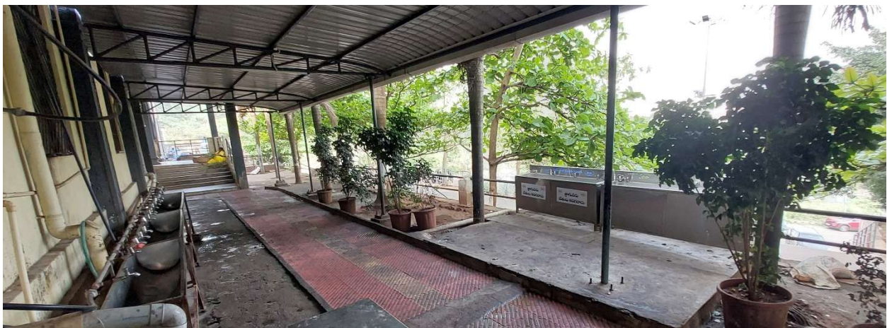
Pic 3 - Handwash and drinking water sinks on opposite sides at Annadanam
