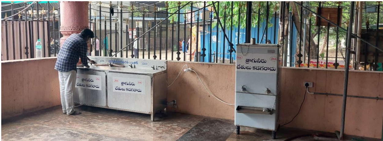
Pic 15 – Chiller and sinks inside the Kalyana Mandapam in Kanipakam
