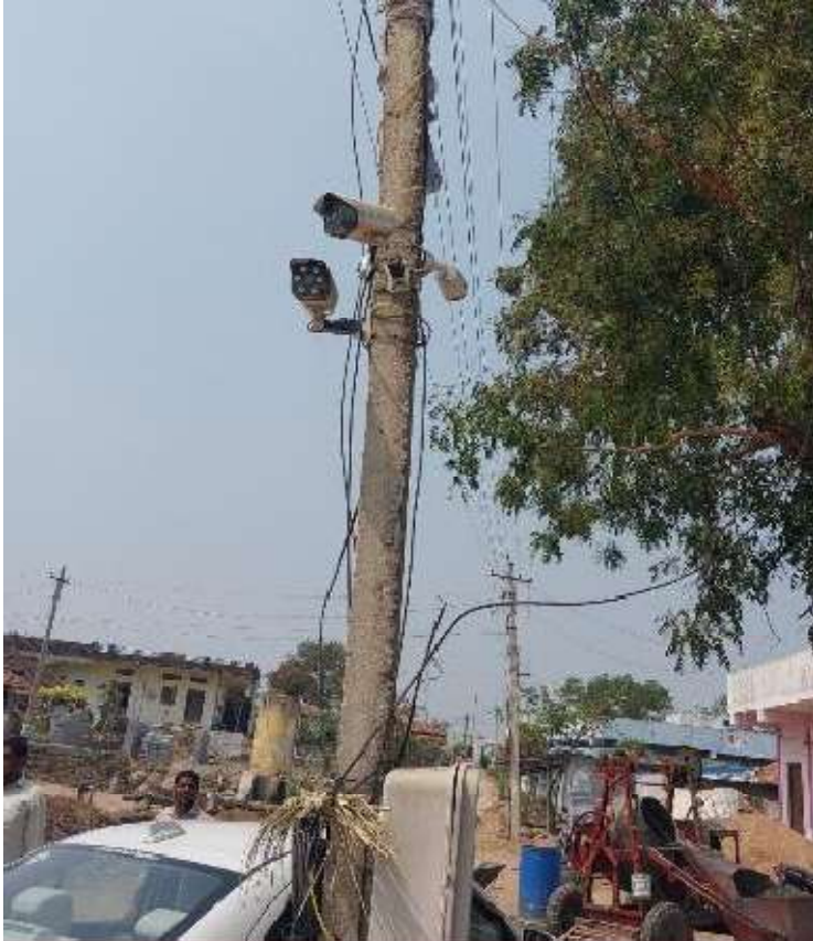
Pic 18 – CCTV cameras installed at Gandhi centre, Gajasingavaram
