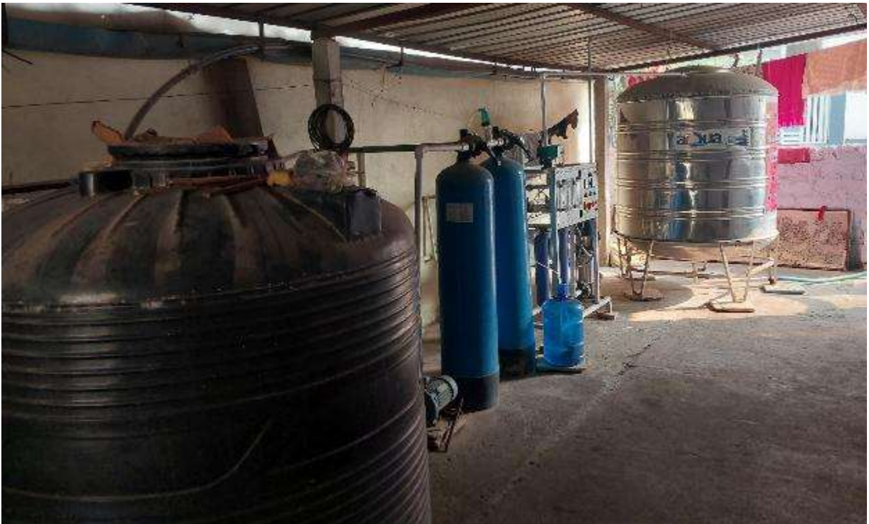
Pic 19 – RO water purification plant installed at MP UPS, BY Nagar, Siricilla
