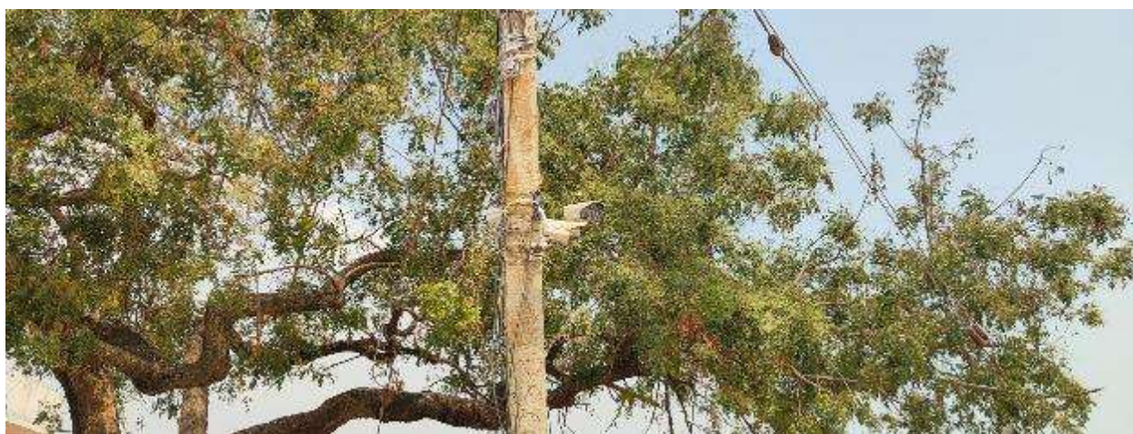
Pic 17 – Closed Circuit TV Cameras installed in one of the locations in Gajasingavaram village
