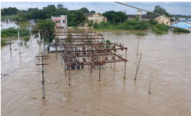
Pic 7 – Power substation submerged in the floodwaters
