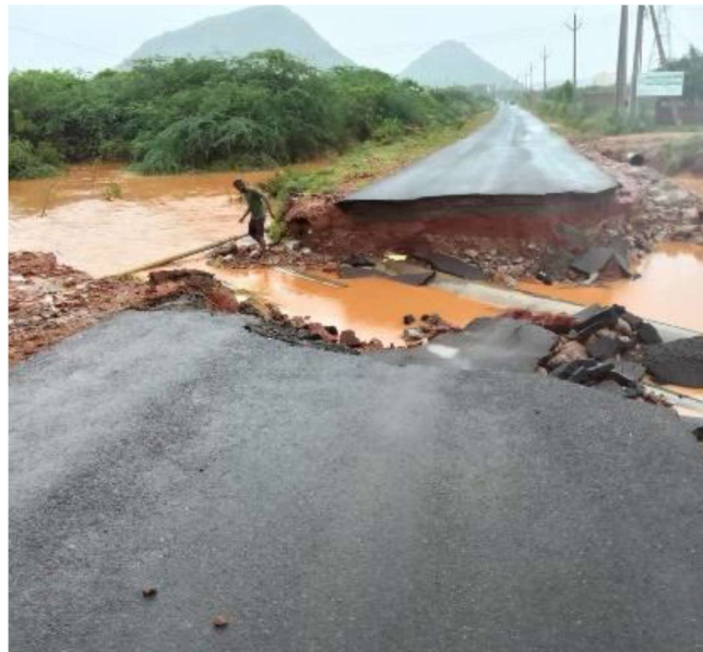
Pic 11 – Road washed away by floodwaters, disconnecting nearby villages
