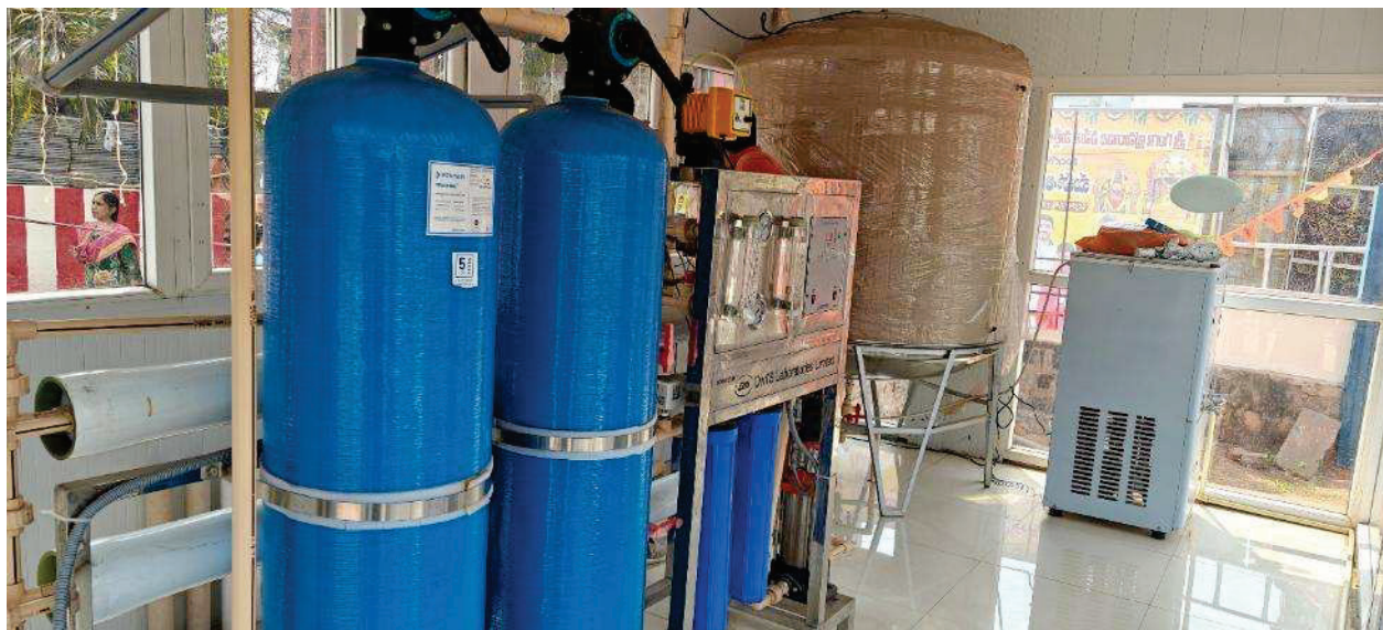
Pic 4 – Interior view of the water purification unit
